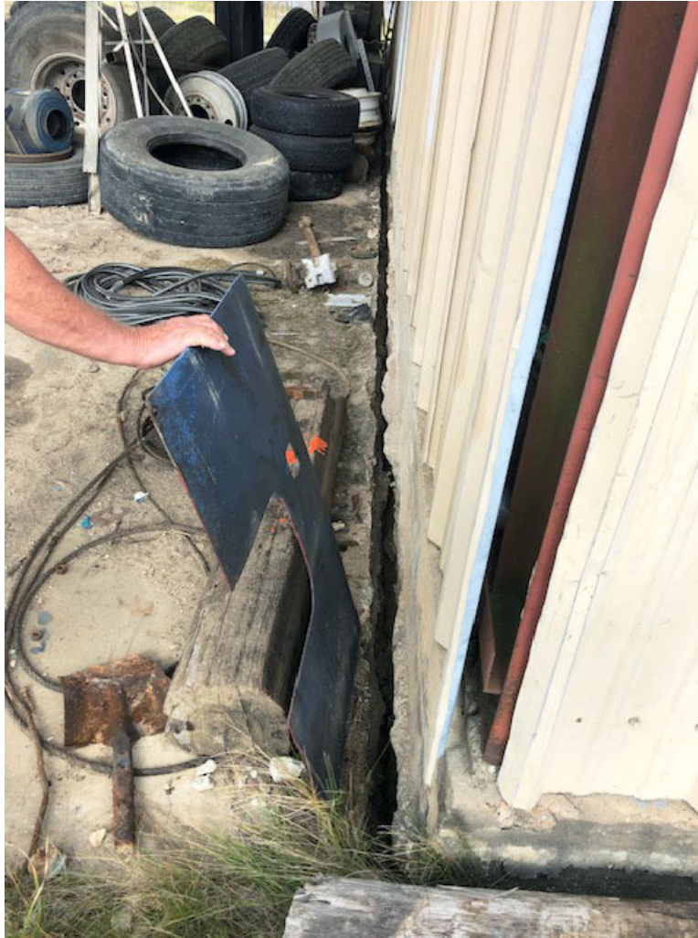
Figure 8. Concrete slab separation beneath a metal-frame building just east of the 2023 collapse area. Photographed on December 10, 2021 by Nat Holcomb. This is the first reported evidence of ground instability within the collapse area of the April 2023 sinkhole.
