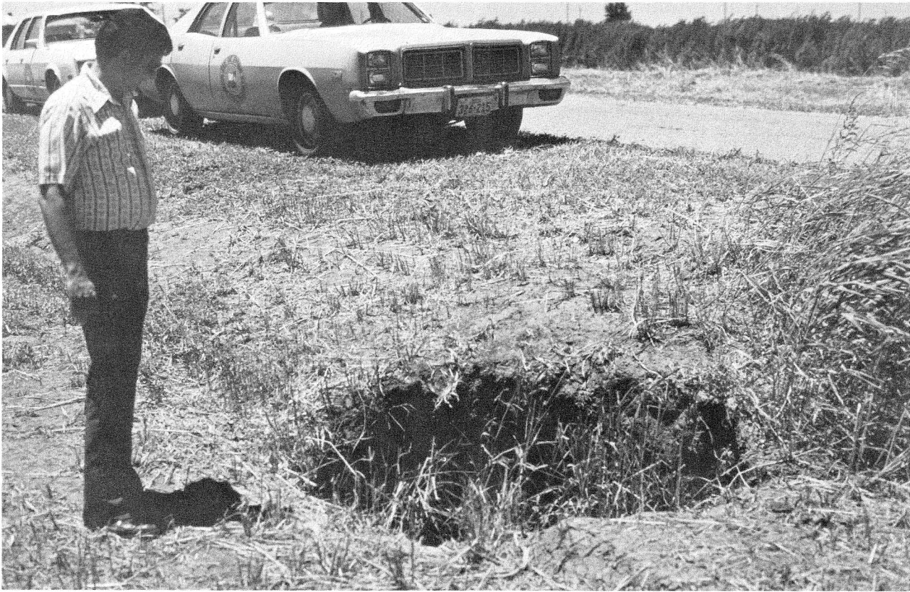
Figure 9. Sinkhole in the borrow ditch adjacent to FM 1034 west of Arlie, Texas. The sinkhole is approximately 0.9 m (3 ft) deep and 1.2 m (4 ft) wide. Sinkholes of this type are common along highways in the Texas Panhandle.
