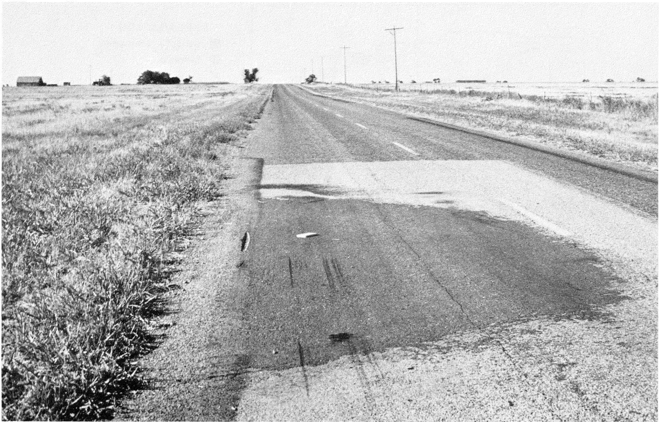
Figure 8. View south along FM 1033 in Childress County showing collapse depression. The depression affects most of the northbound lane and extends into the borrow ditch. Different shades of road patches at this site attest to the history of subsidence.
