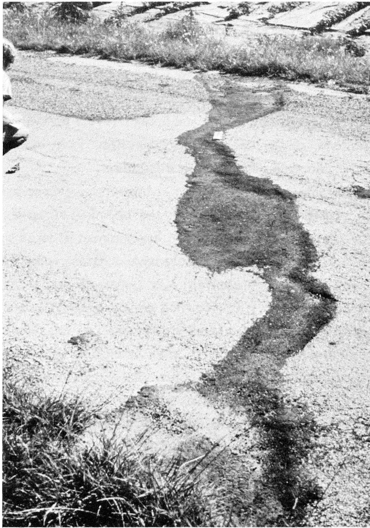
Figure 10. Fault trending northeast across FM 2639 in Hall County. Left side of fault is depressed approximately 3 to 4 cm (1.5 to 1.8 inches) relative to the right side. Fault extends into the cultivated field.
