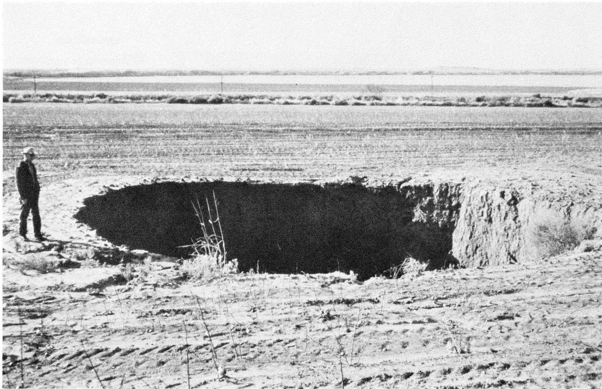
Figure 5. Sinkhole located near U.S. Highway 287, 6.4 km (4 mi) northwest of Estelline in Hall County, Texas. The feature is approximately 10.6 m (35 ft) wide and 7.5 m (25 ft) deep.
