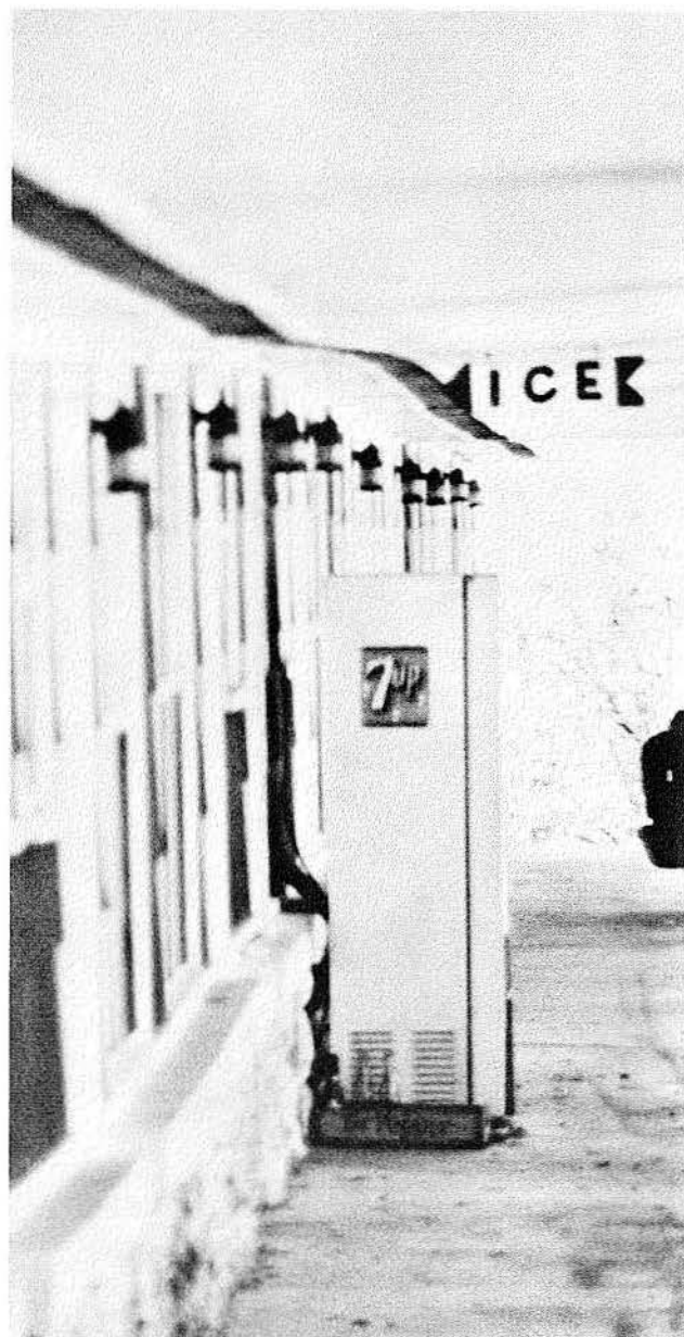
Figure 12. Microridge development (in the area of the soft drink machine) resulting in extensive damage to concrete walks, drives, stone facing, and interior walls of this motel
