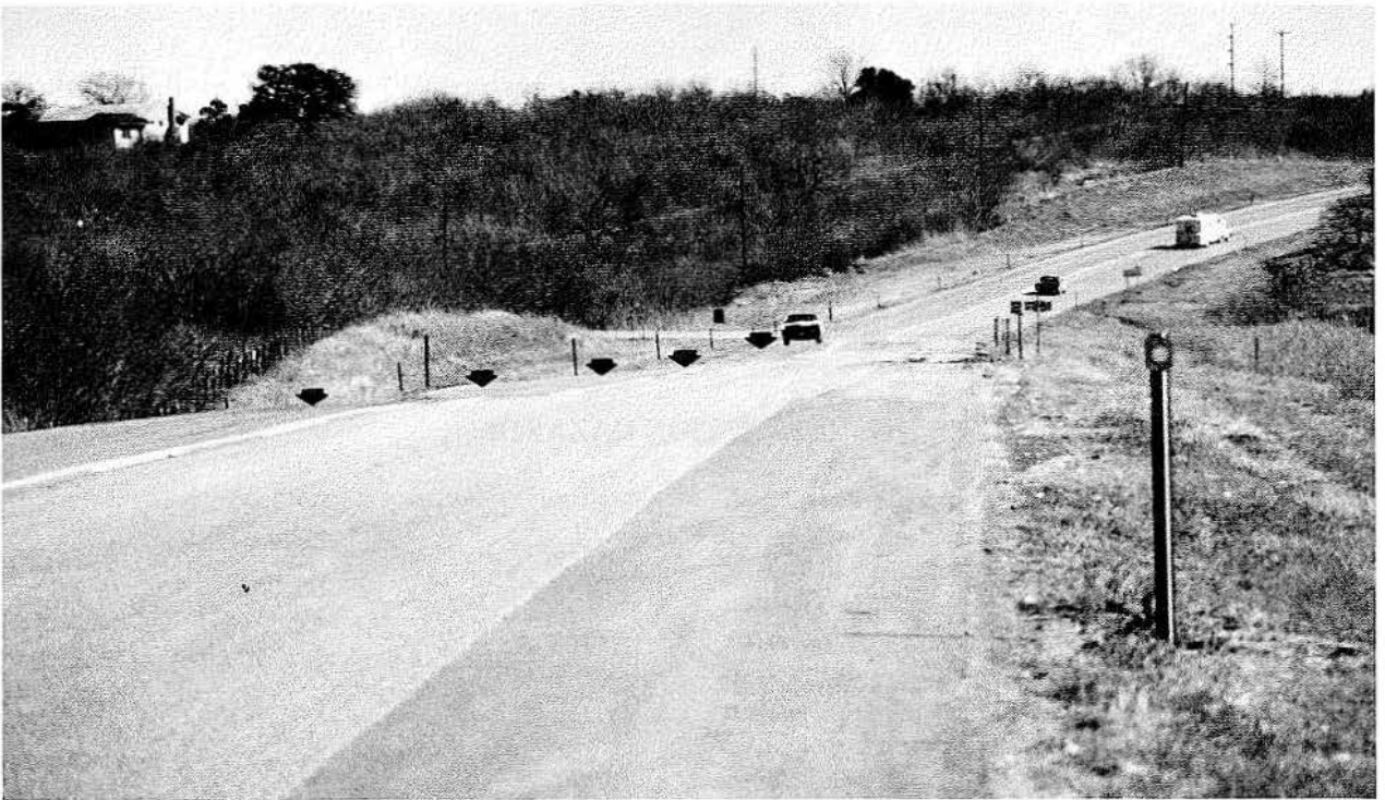
Figure 13. Rippled road surface and cracks on U. S. Highway 183 north of Gonzales, Texas
