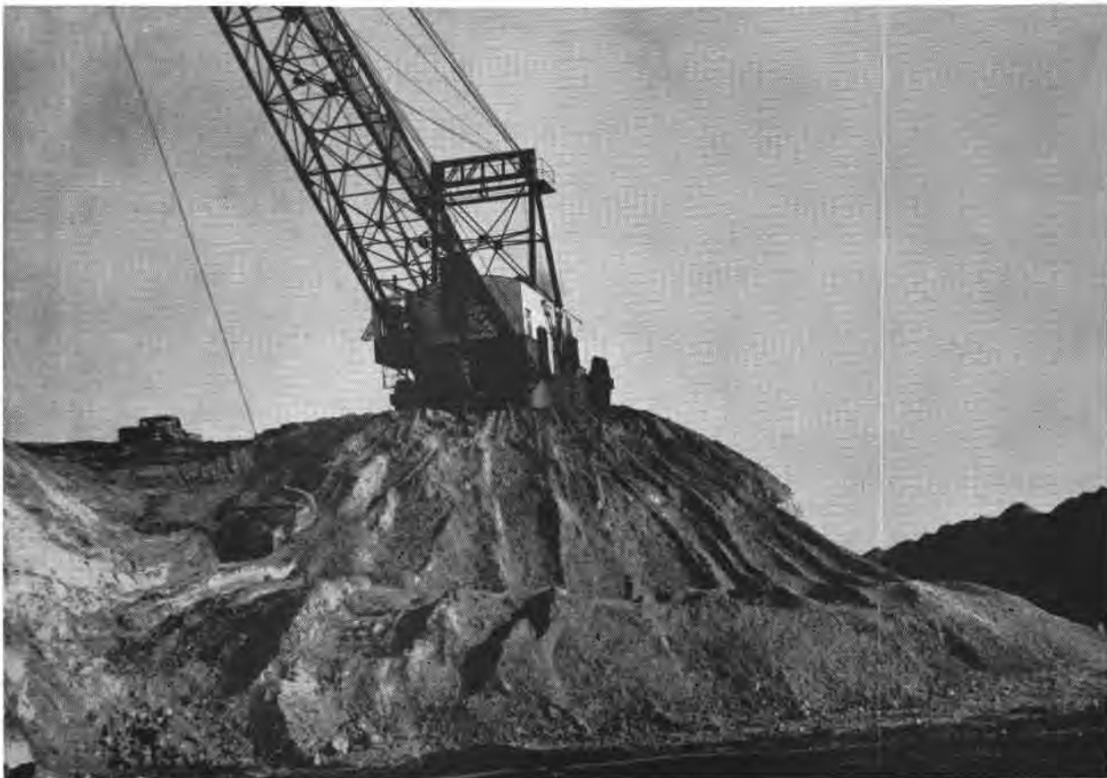
Dragline stripping at the Darco lignite mine of Atlas Chemical Industries, Inc., Harrison County, Texas. September 1962.
